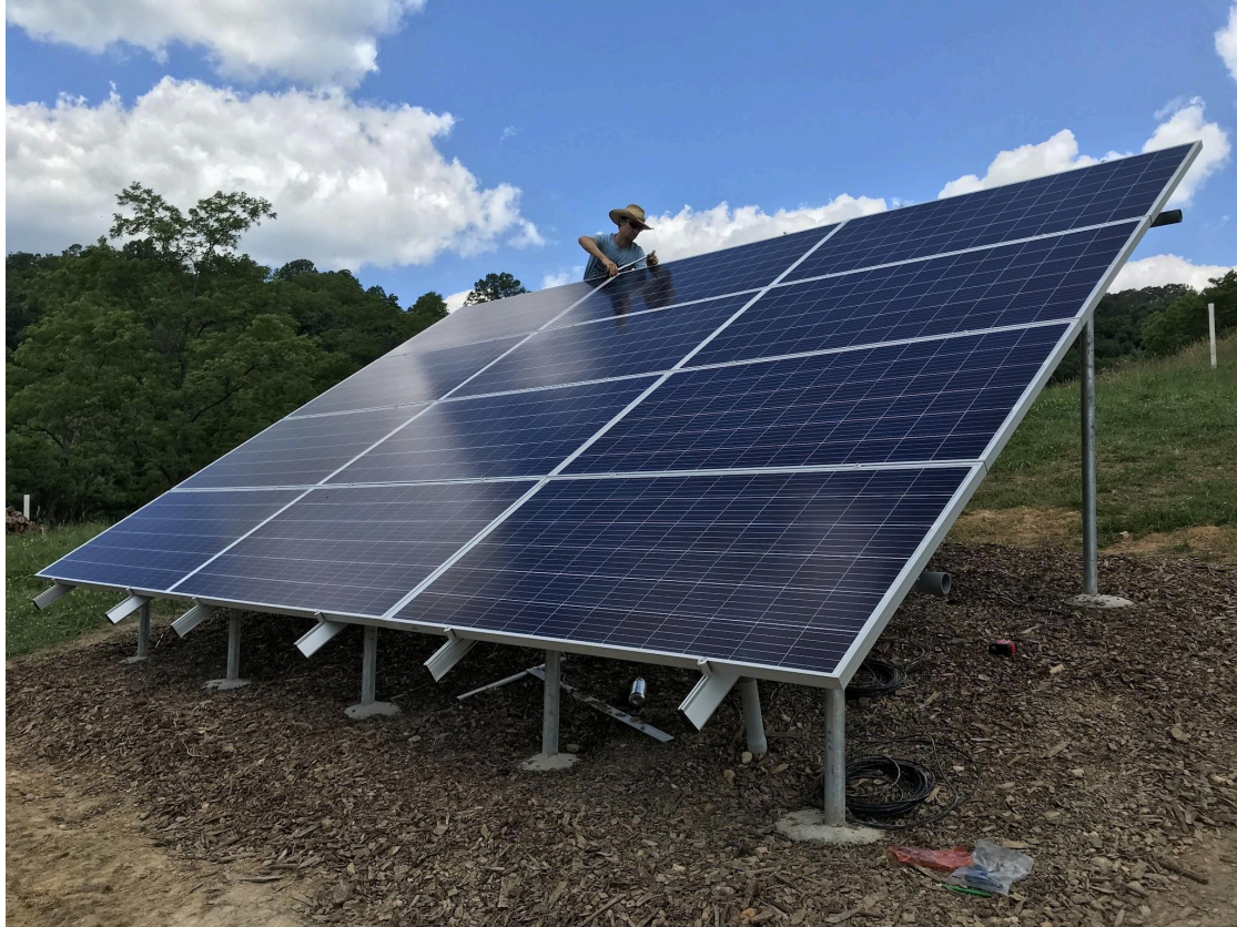
Solar panel array
